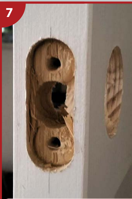
7. Example of 'door preparation' completed - ready for the latch/bolt to be installed.
